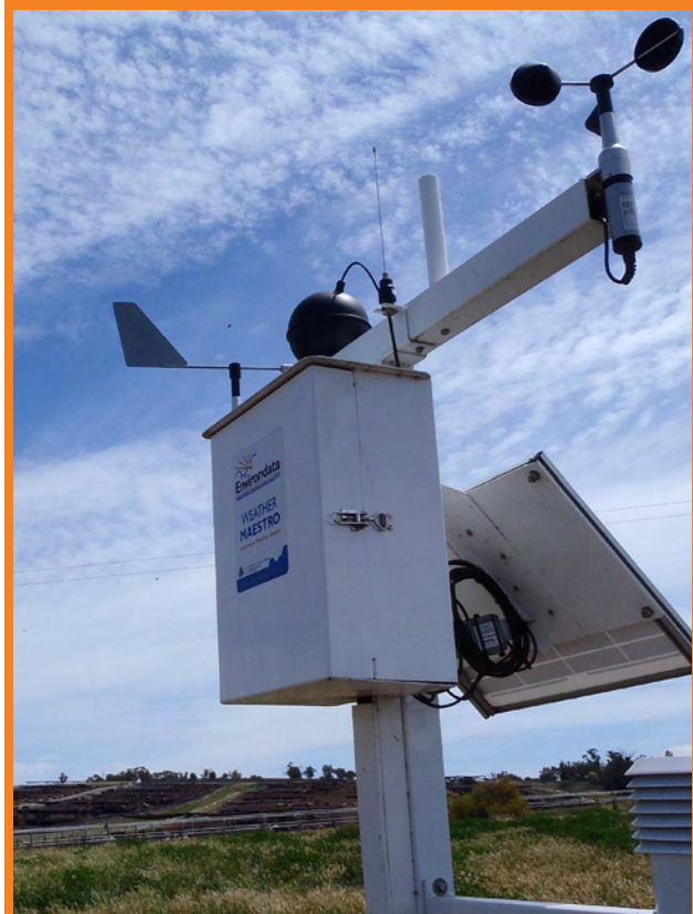
Weather Maestro with UHF link installed 2010
